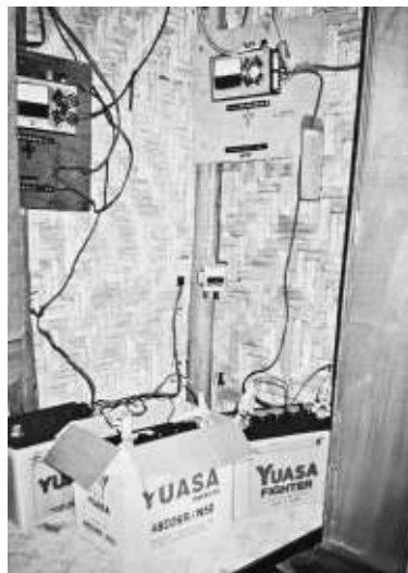
Batteries and transformers
